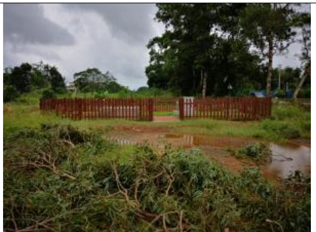
2号污水提升泵 (E110° 32' 59.70567" , N19° 43' 52.62078" )
