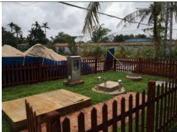
1号污水提升泵 (E110° 34' 4.55505" , N19° 42' 22.39556" )
