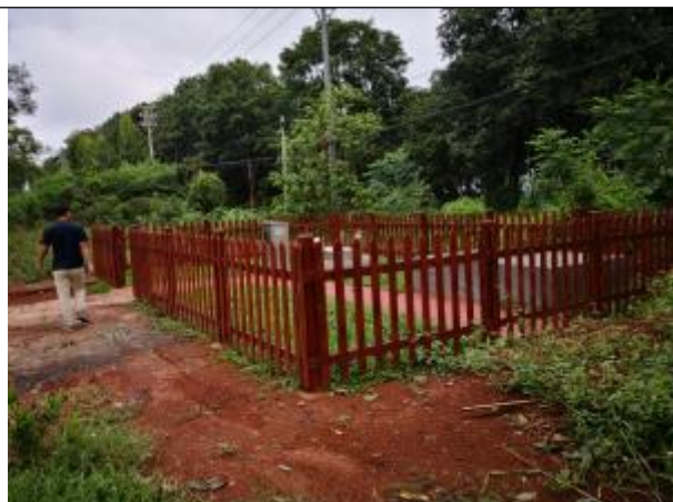
3号污水提升泵 (E110° 32' 56.98746" , N19° 44' 14.31635" )
