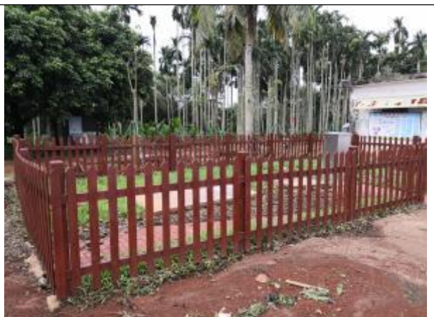
红明大道污水泵站 (E110° 32' 29.71905" , N19° 43' 38.43483" )
